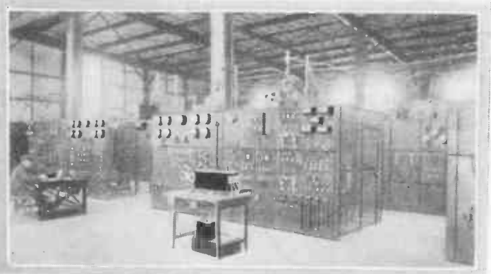
This photograph shows a portion of the stupendous installation of equipment used at the Rocky Point, L. I., station. When it becomes possible to carry on a radiophone communication with foreign countries, it is said that the charge for a 3-minute conversation to London will not exceed $5.
