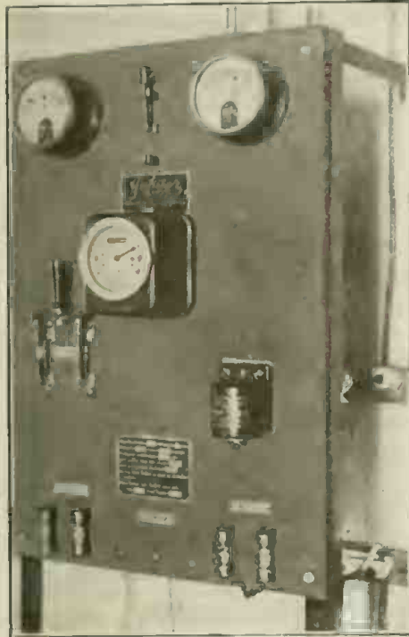
Appearance of Automatic Electric Switch-board Used in Wind-power Electric Plants. It Cuts in the Dynamo When the Wind-mill Has Attained the Proper Speed.
