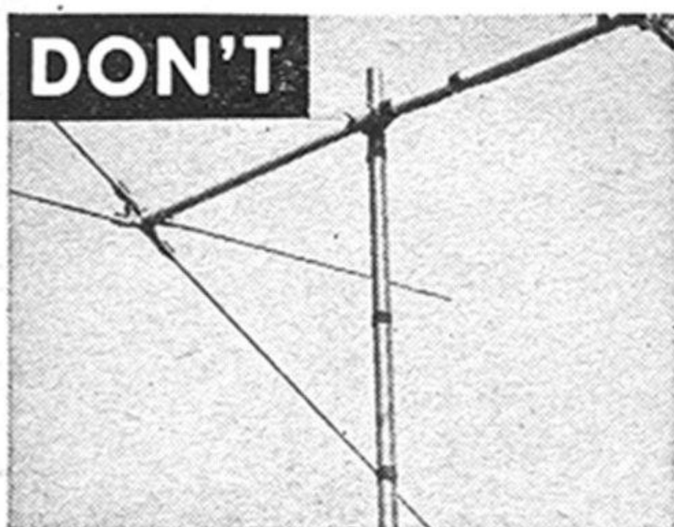
DON'T ... Fasten a lead-in tightly to a mast this way. Use stand-offs.
