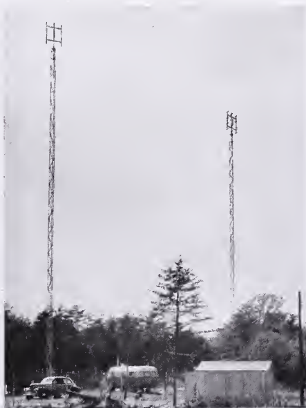
FIRST LINK in the Philco network, at Arlington, Va., uses 100-foot dipole-topped antenna towers for line-of-sight transmission.
