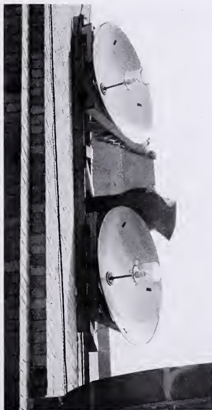
PTM receiving and transmitting antenna installation atop IT&T Building, New York.
