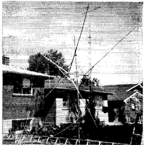
A dry run near the ground to insure that everything will fit together properly when the antenna is permanently installed.
