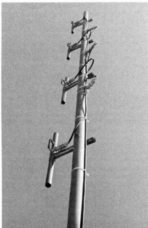
Collinear antenna with elements placed for skewed pattern. Gain in this configuration is approximately 9 dB. Note placement of harness away from elements.
