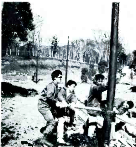
Construction of distribution facilities also involves a great deal of manual labor.
