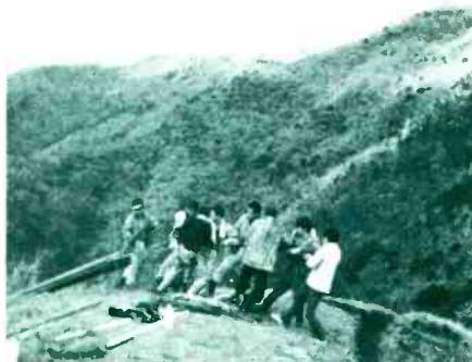
Poles for antenna mounts and trunk run down the mountain are transported and installed by hand.
