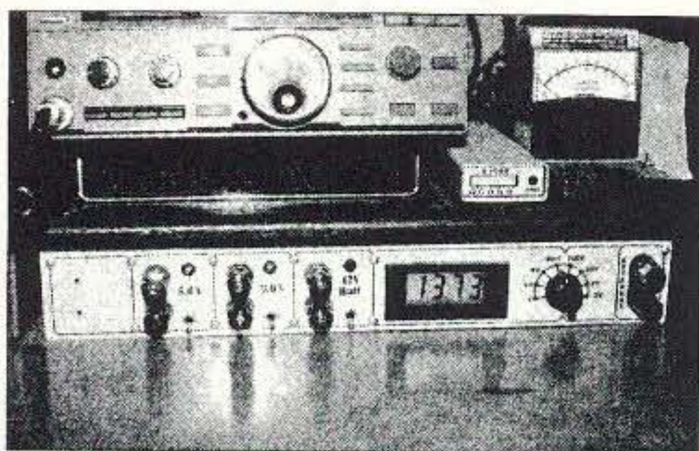
Photo A. Power panel in its operating location.
