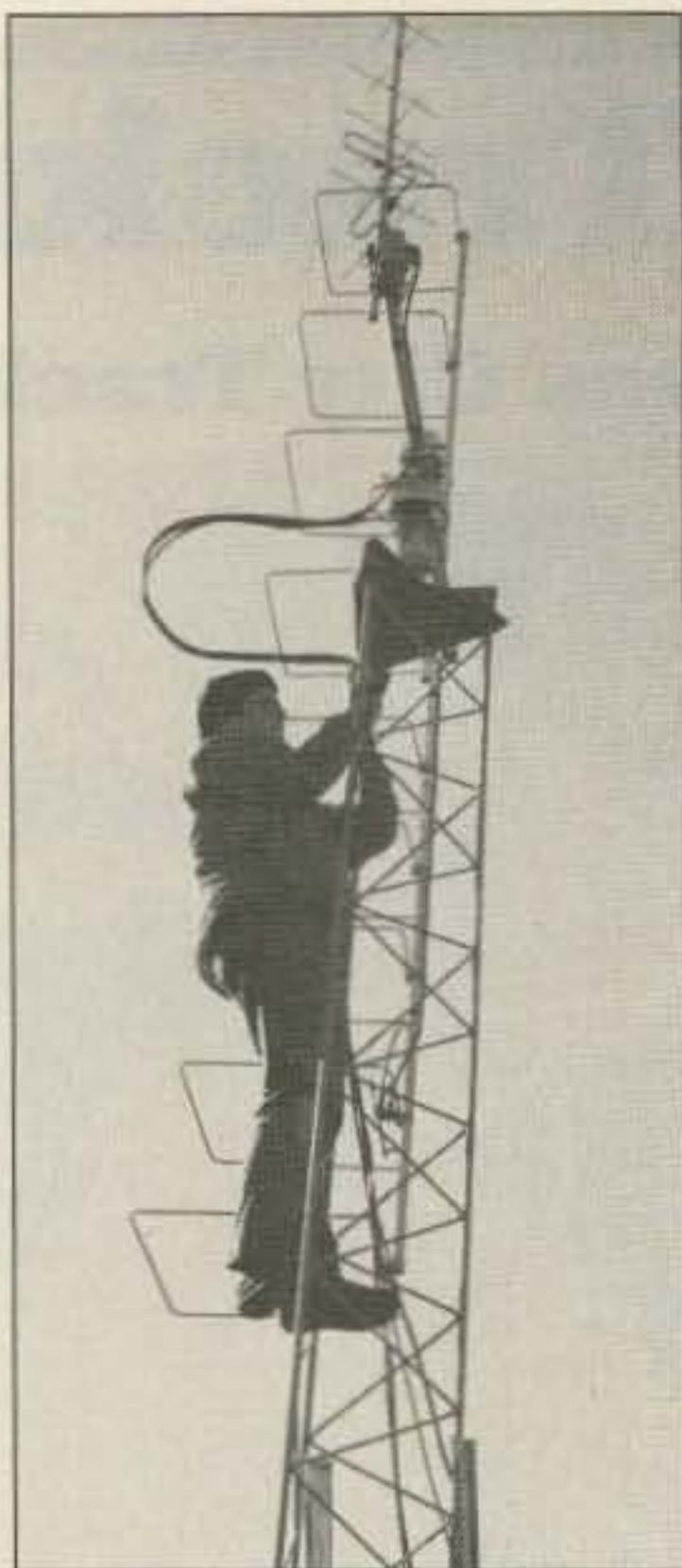
Photo C. WA5ZIB puts a generous loop in the feed/rotator lines from the antennas to the tower.
