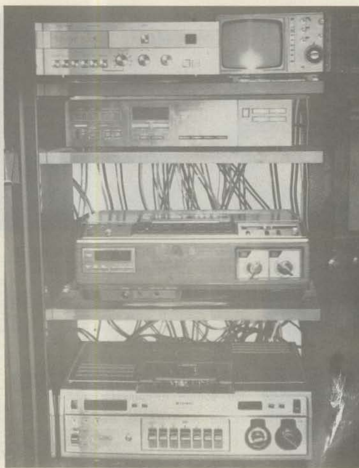
Photo H. The video rack with Drake receiver, Pioneer video tuner, and two Beta video cassette recorders.
