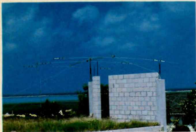
Once atop the wall, the antenna was tied off to prevent the ever-present tropical breezes from tearing it to pieces. Kansas is dead ahead.
