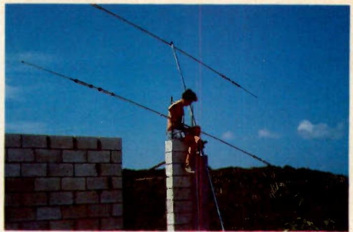
A partially-completed cinder-block wall provided a sturdy support for our tribander. Here, Tim prepares to hoist the antenna into place on a protruding piece of reinforcing rod.
