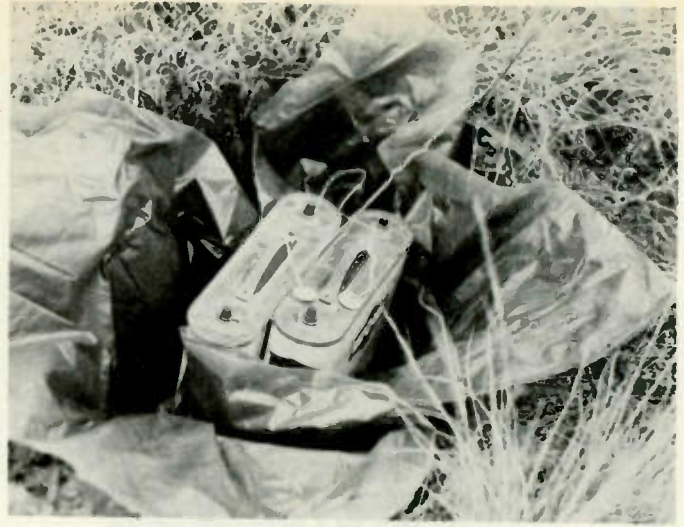
Photo C. The batteries for the transmitter.
