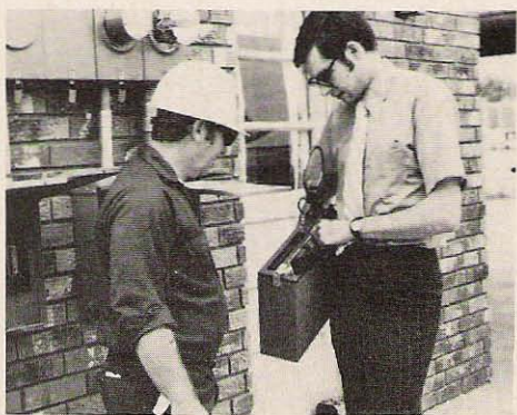
The first place to start is at the main breaker panel of the house experiencing the trouble. Here the author is working with a power company serviceman to locate the noise.
