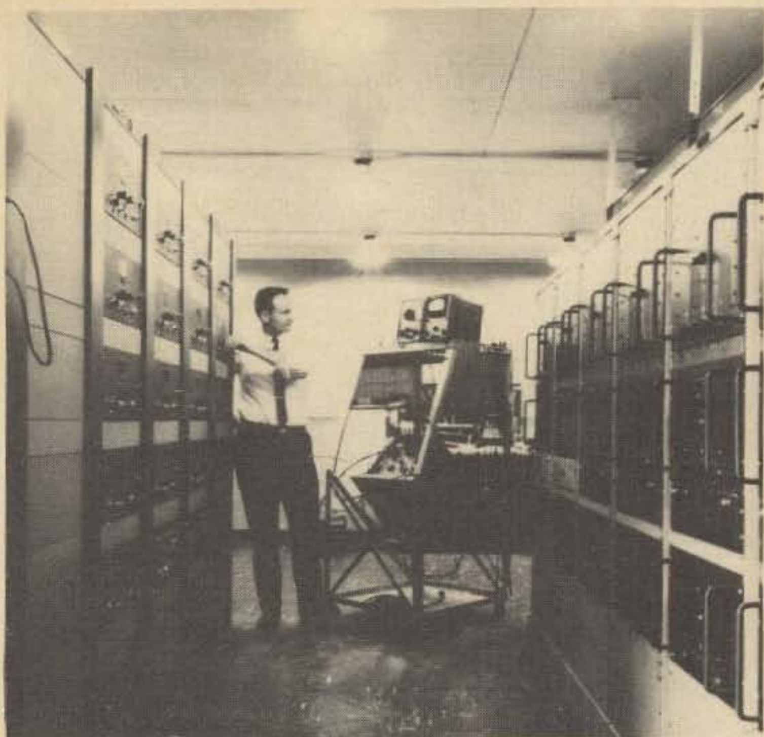
FAA Field Service Technicians aligning UHF receiver banks. In addition to on-the-job training, the FAA provides excellent classroom instruction at the FAA Academy.
