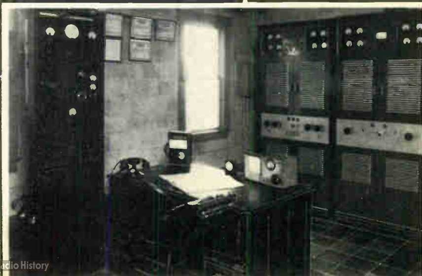
The Main Transmitter Room at W9XBY. Here you will watch and record the operation of this ultra-modern 1000-watt transmitter.
