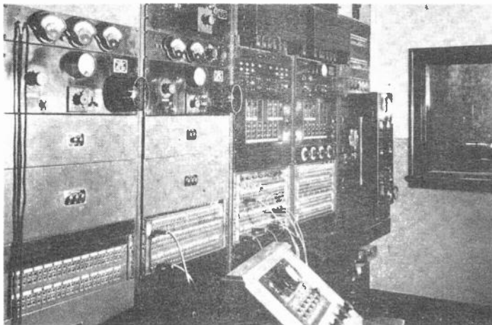
Fig.1 Control room of station KMBC.
