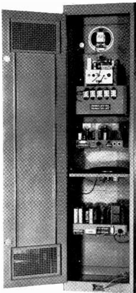
Complete p-a assembly showing monitor speaker at top, below which is the radio tuner, amplifier, phono turntable, and power supply.
