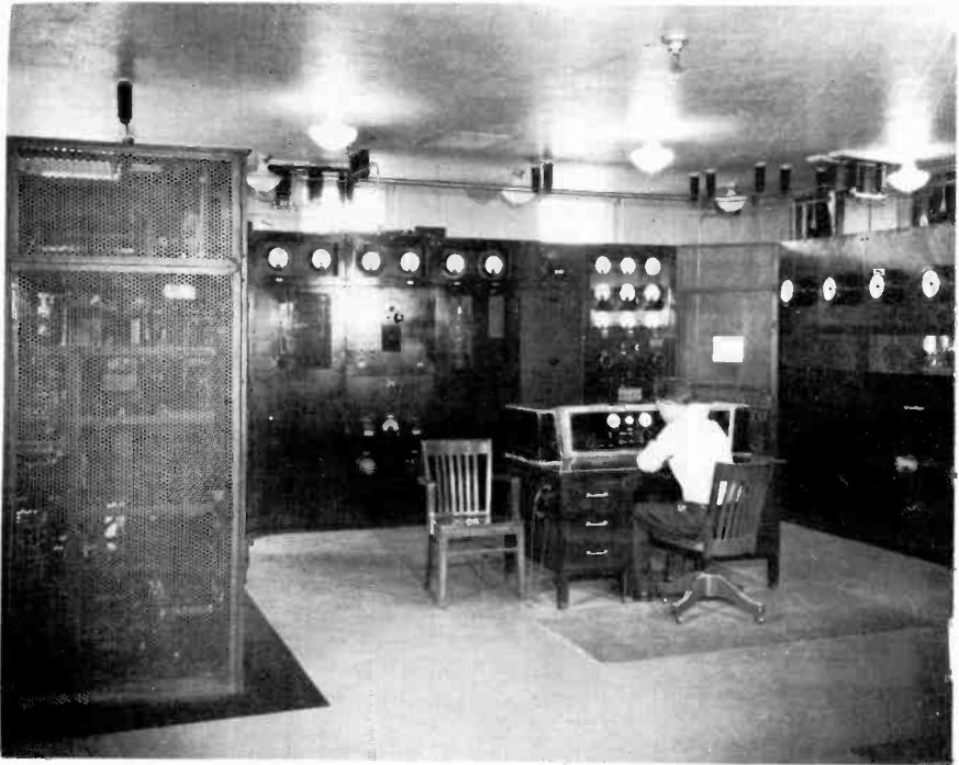
Transmitter room showing equipment and control desk.
