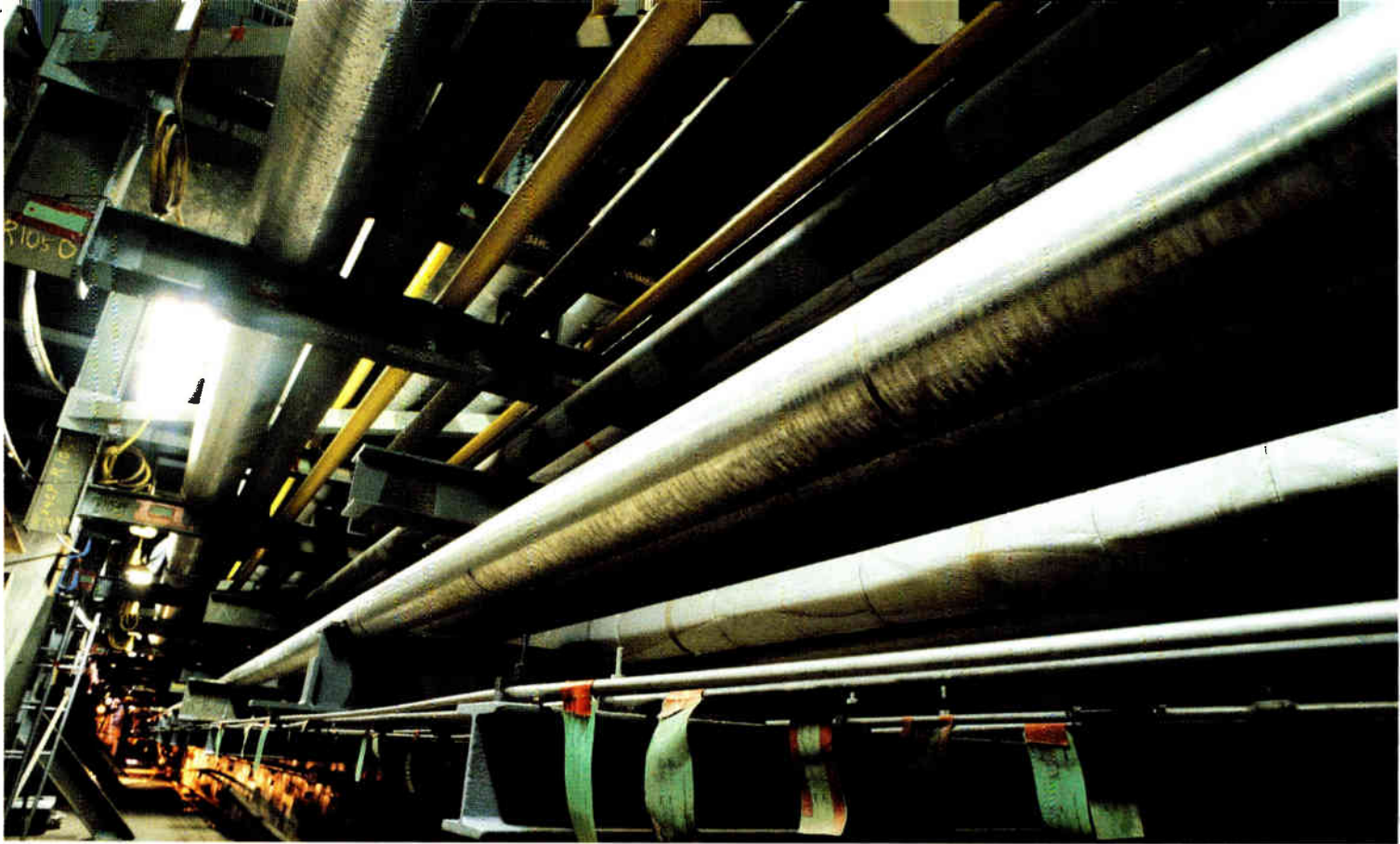
3—Section of piping in nuclear plant.
