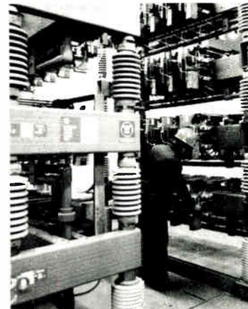
VAR generator controls
