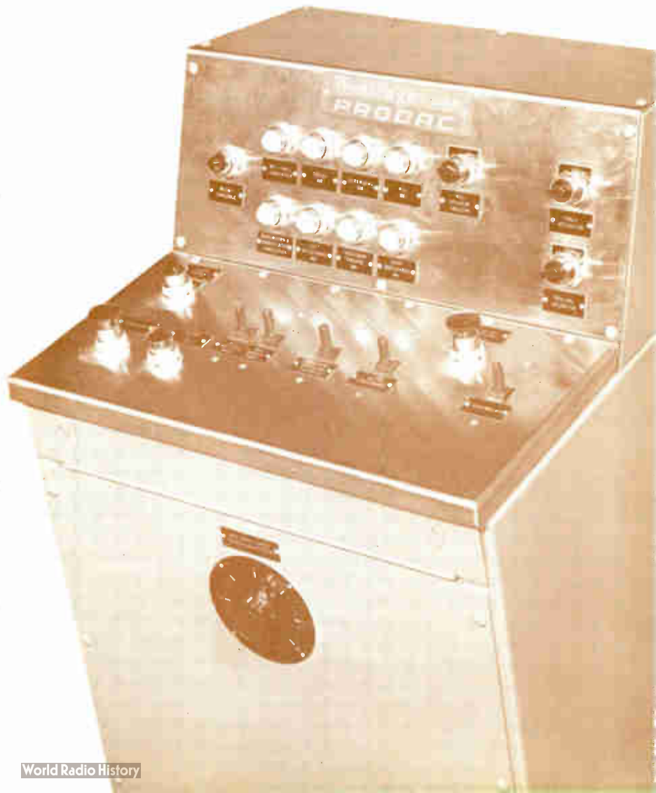
Fig. 5—Manual take-over control for blooming mill using small master switches.
