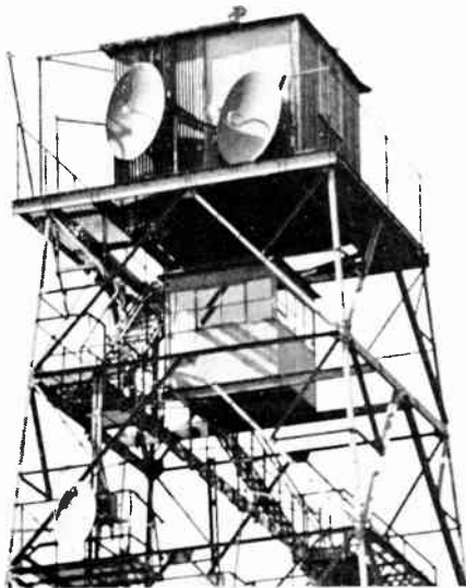
Figure 5. New horn-fed antenna unit mounted adjacent to old type unit
