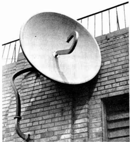
Close-up of horn-fed antenna unit
