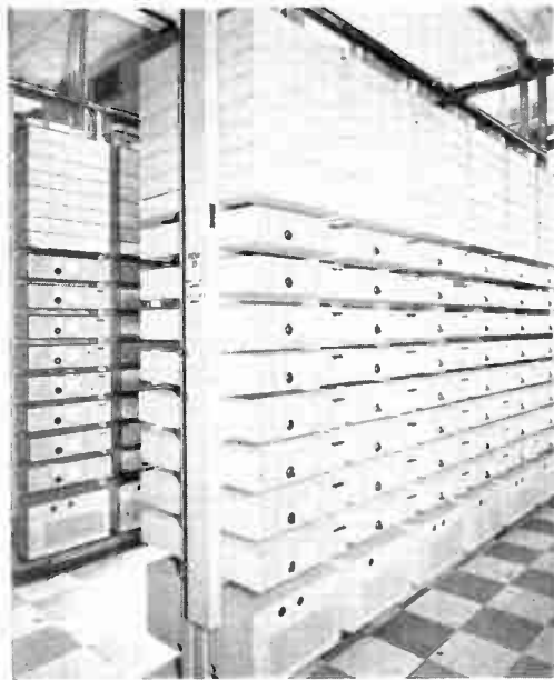
Figure 1. Channel terminal equipment in large office
