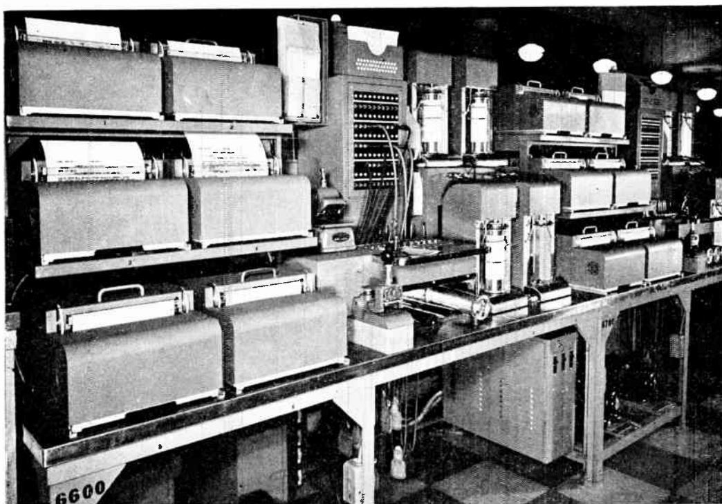
Figure 5. Two-table Desk-Fax concentrator installation at New York
