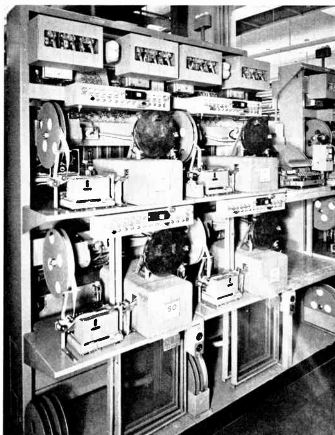
Figure 39. Line receiving positions for heavily loaded tributary and branch office circuits—Type 4930 racks
