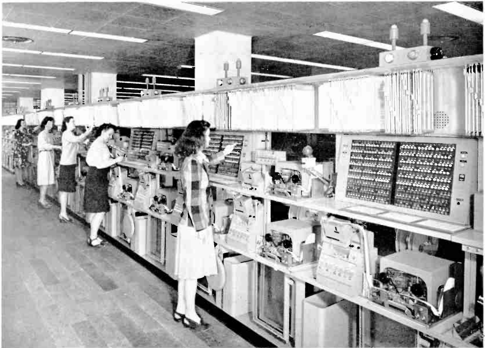
PUSH-BUTTON SWITCHING INSTALLATION AT PHILADELPHIA, PA.
