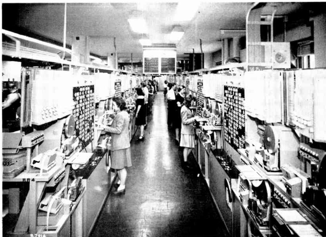
Figure 3. Main switching aisle—St. Louis, Mo.
