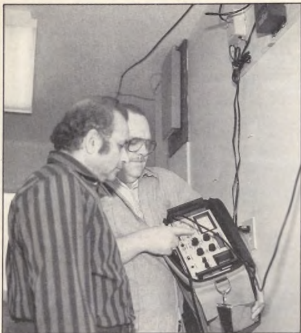
Fig. 4: Mr. Patel, the manager of the King's Inn Motel, watches as Walter runs through a 6 month system checkout to keep every room's picture at top performance.
