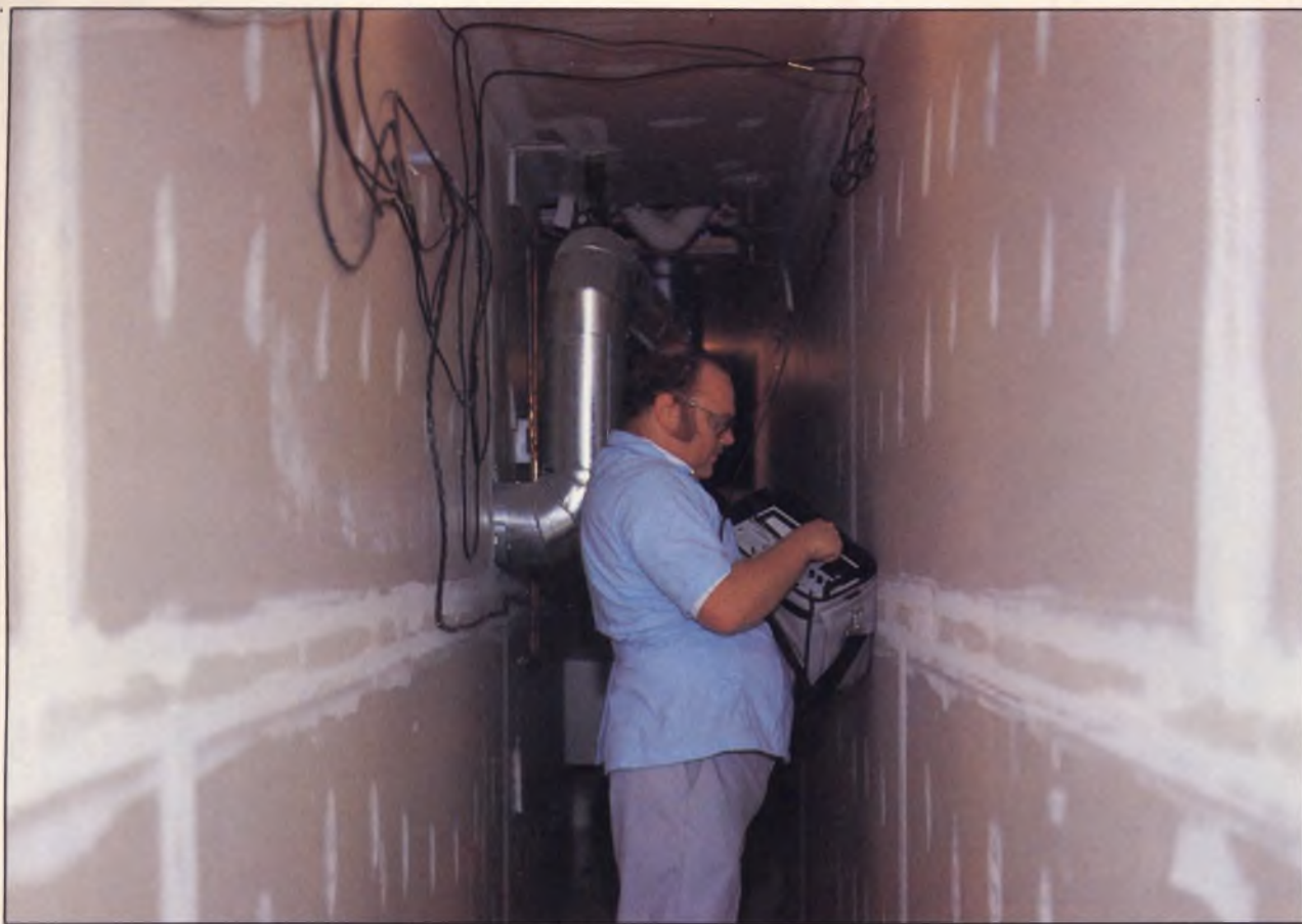
Fig. 2: Nearly half the rooms were dead until Walter found the service hallway in the back. His CHANNELIZER SR. let him fully analyze the MATV signals in the cramped quarters.
