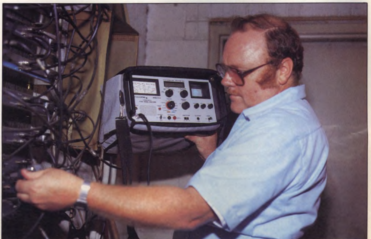
Fig. 3: Balancing the strip amplifiers in the hospital headend restored clear pictures, even in the most distant room.
