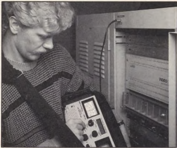
Fig. 3: Independent miniature cable systems offer servicers new opportunity. Above, signal levels are being checked in a motel cable system.
