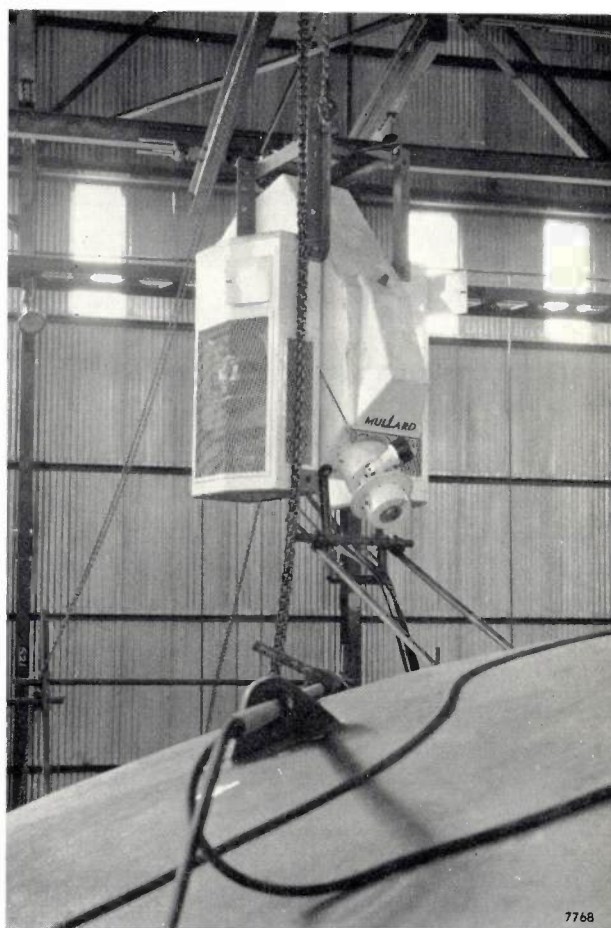
Fig. 1. 4 MeV industrial radiography installation, equipped with a linear accelerator (Mullard), in operation for examining the welds of one of the pressure vessels under construction for the nuclear power station at Trawsfynydd, North Wales 9) . (Photograph by courtesy of Atomic Power Constructions Ltd.)
