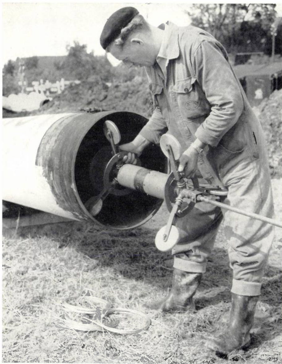
Fig. 11. Application of the gamma rays from a radio-isotope (iridium-192) for radiographing the welds in a pipeline. The holder with the radiation source is introduced into the pipe on a kind of trolley and pushed to the site of the weld, where an X-ray film is laid around the pipe. The source is operated and the film exposed by remote control. (Photograph by courtesy of "Röntgen-Technische Dienst", Rotterdam.)
