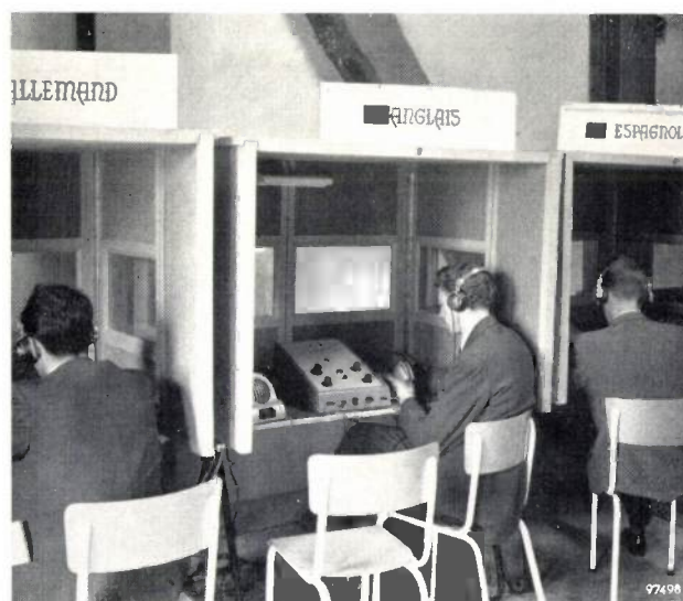
Fig. 5. Interpreters' cabins of the simultaneous interpreting installation in the Grand Auditorium at the 1958 Brussels Exhibition.
