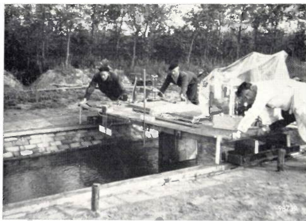
Fig. 5. Bridge with detector and instruments, used for the preliminary experiment at the De Voorst hydrological laboratory.
