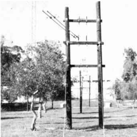
View of H-Frame, Showing Transmission Line Leading to Antenna
