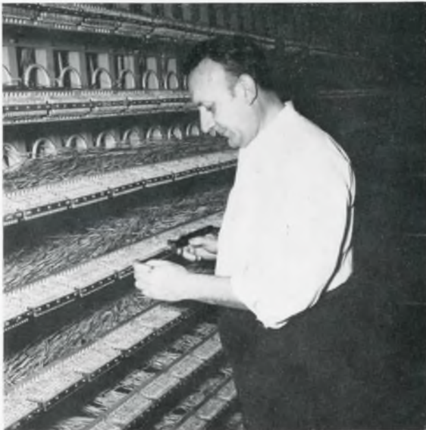
SOLDERING WIRES on terminal equipment in Plant 2 is one of the duties of Frank Lodge of the Bell Telephone Company, who has charge of moving and installing new telephones in the Philco plants.
