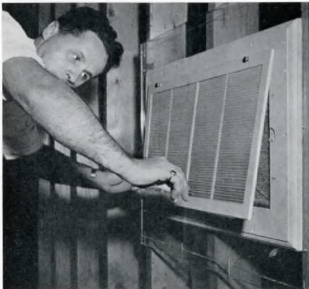
FINAL INSTALLATION of the return air grille used in Philco's "do-it-yourself" kit. A permanent type aluminum filter is used. The filter requires only washing and spraying with an aerosol oil mist to renew its filter action.
