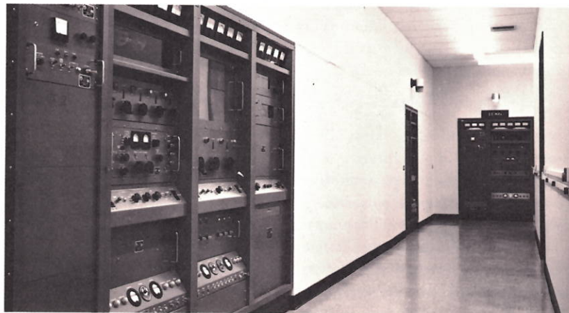
Figure 7—WWV's 15 MHz TMC Model GPT-40K, a Transmitter which Uses the Forced Air Cooled ML-6697 or ML-6697A.
