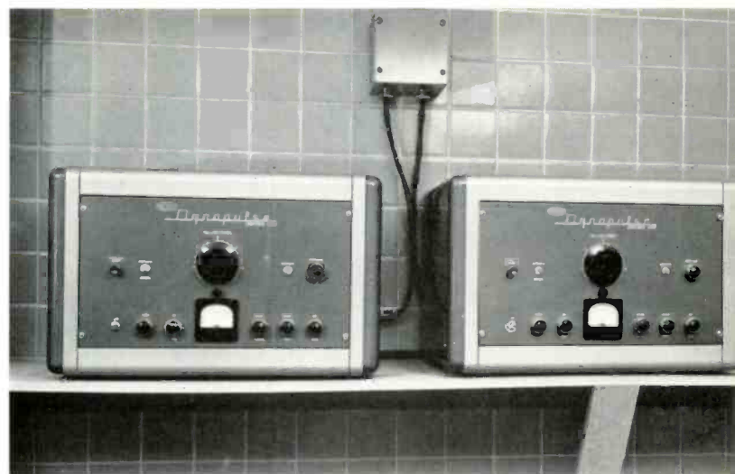
Figure 1 — The dynapulse control panels are mounted in a position reasonably accessible but not necessarily in the technician's control area. They are used only to preset the millisecond timing and are not needed for initiating the actual exposure.
