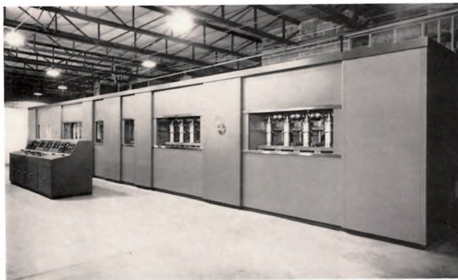
Figure 4—General view of the front panel of the megawatt transmitter and the centralized control console.
