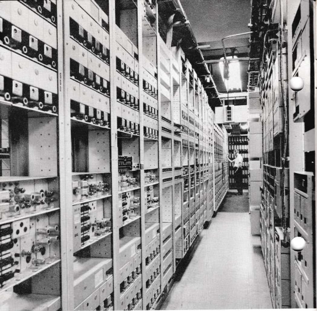
Figure 1. Lenkurt 45BX carrier equipment in telephone toll center. Protruding equipment on right is Lenkurt 33A carrier, a classic older design still in great demand because of its reliability and performance. Relatively controlled environment in such centers reduces an important problem forced on military equipment.
