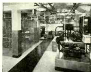
Power room at WJR, Detroit.
