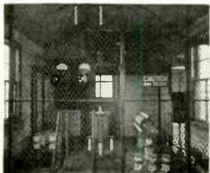
Antenna coupling equipment.
