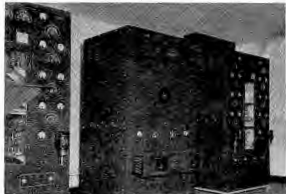
Right, dual radio-range transmitters and coupling unit, in center, at South Pacific project.
