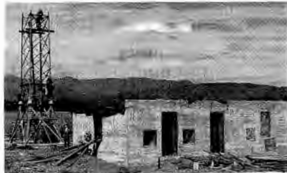
Right, above, excavations for tower footings at South Pacific radio-range project. Right, a splinter-proof (bomb-proof) cement building to house the radio-range equipment on a South Pacific island.
