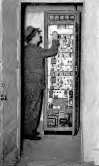
REMOTE STATION HOUSING TRANSMITTER AND DUAL RECEIVERS AT BASE OF ANTENNA TOWERS
