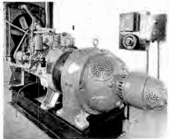
Figure 9 The gasoline engine, alternator and exciter that was selected by chief engineer Karl Troeglen as an emergency power unit for station WIBW.
