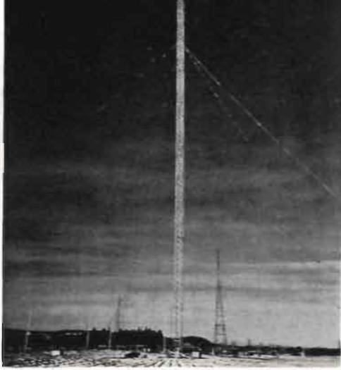
The 625-foot tower at General Electric's station WGY, Schenectady, N. Y., under construction by The American Bridge Company.
