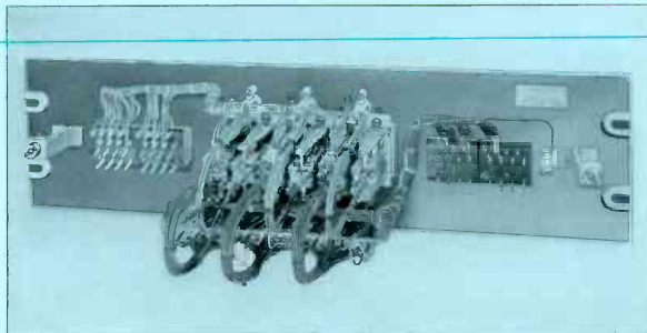
REAR VIEW OF THE 270A OUTPUT SWITCHING PANEL
