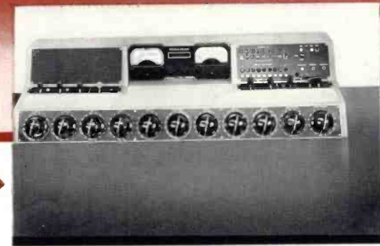
Main control panel showing convenient placement of frequently used controls and indicators directly in front of the operative engineer and in line with his vision into the studio.
