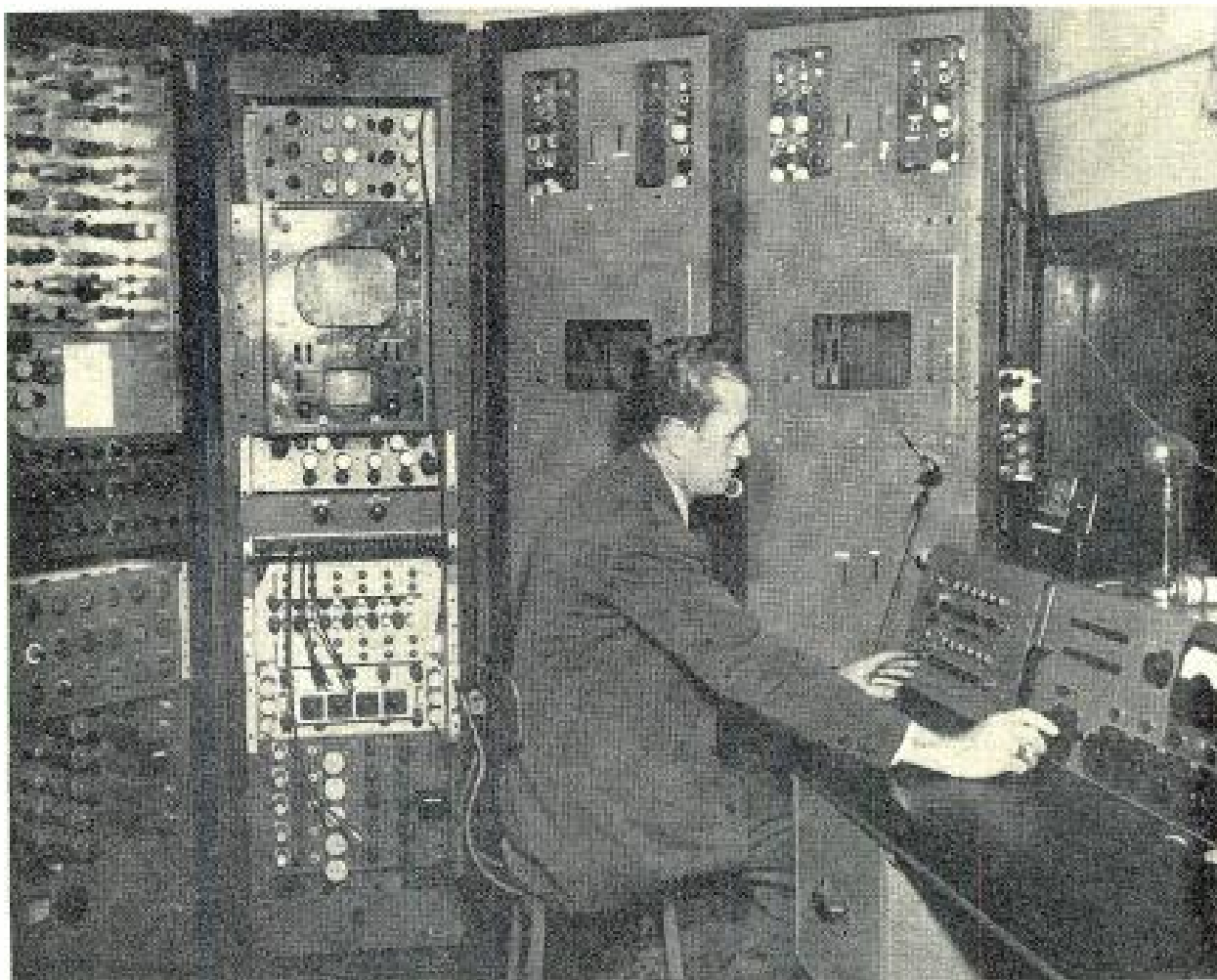
Fig. 3 — Experimental color television equipment installed in the control room of the Wardman Park studio.
