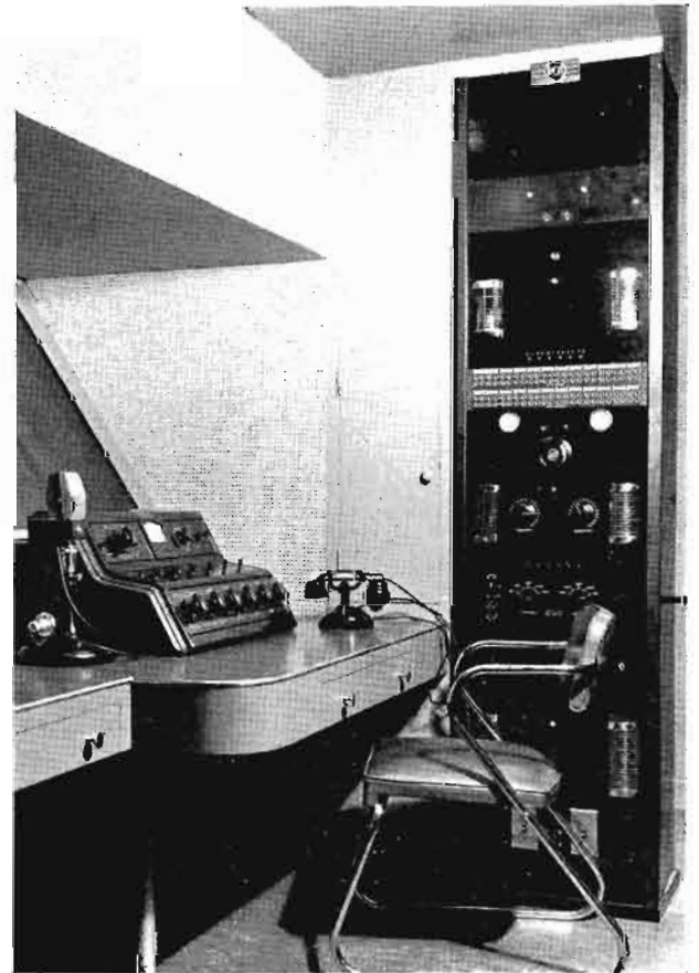
The RCA 78-C Equipment in the Control Room of Studio 2 at Columbia's WCCO.
