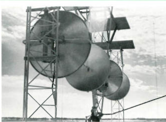
WBAP - Fort Worth - WFAA - Dallas. Isolation techniques on 3-tower Directional AM Northlake Texas site. WBAP, 50 KW Non-Directional, WFAA, 5 KW DA-2. Sharing same antenna system. Both with "Hot Standby."
