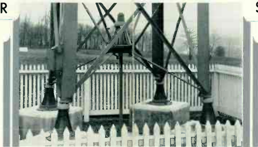
Low Capacity Insulator Arrangement—the Outstanding Feature of the Blaw-Knox VERTICAL RADIATOR
