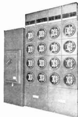
Over-6-circuits Grouped Metering Equipment
