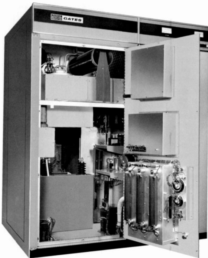
Modulator cubicle, showing modulator, modulator driver, 70 kHz filter, power supplies and control.
